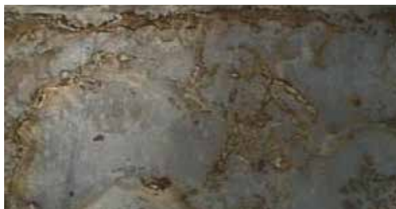
Fig. 1.3.4 Poor rinsing, material stored wet
