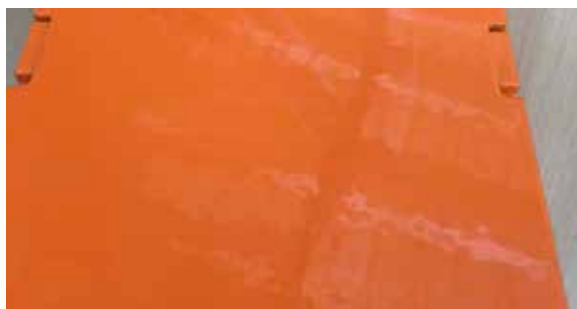
Fig. 4.9.1 Effet efflorescent (blooming)
